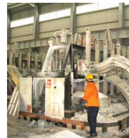
14 November, 2012 The initial commissioning phase of Press Metal Bhd's aluminium smelting plant in Samalaju Industrial Park
