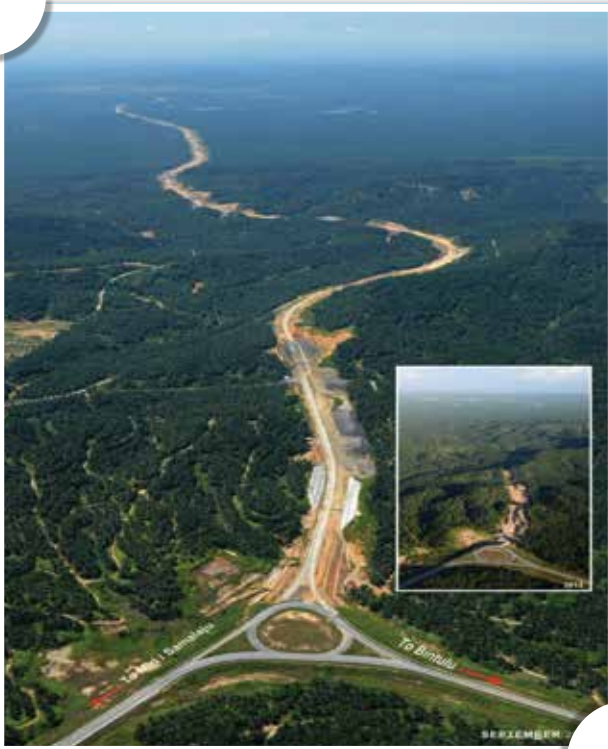
Completion of Mile 32 Road connecting to the Pan Borneo Highway, Bakun HEP and Murum HEP.
