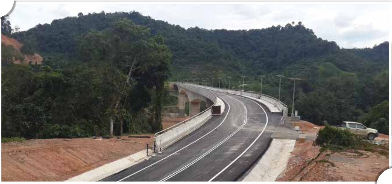
Completion of Baleh Bridge in Kapit Division leading to Tunoh Growth Node and Baleh HEP.
