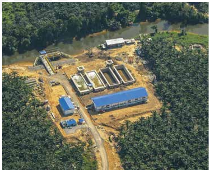
Phase 1 Stage 3 Raw Water Intake at Sungai Similajau
